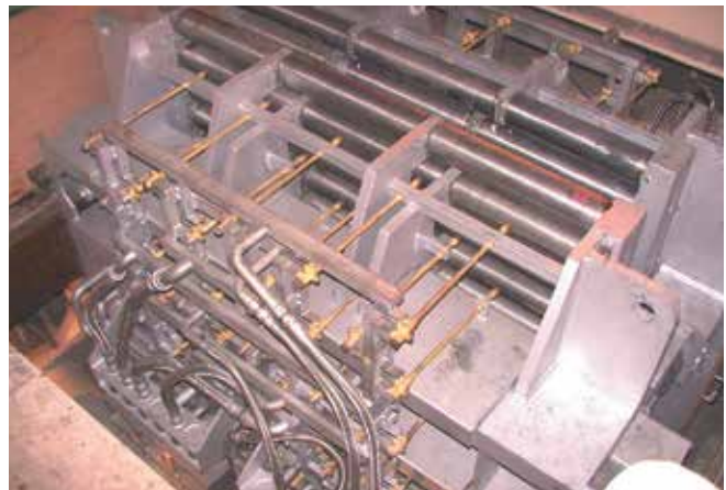
Example of staggered nozzle positions with Mastercooler SMART piping
