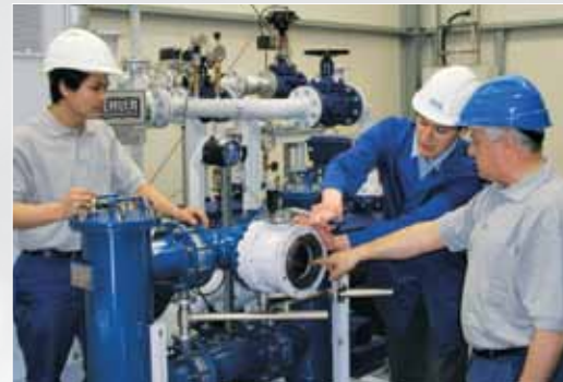
Commissioning and training by Lechler staff
