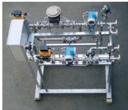
Regulation unit with wiring to terminal boxes
