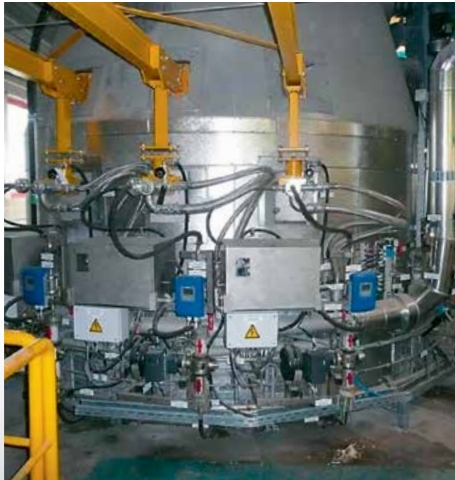
LOC ® reference installation with maximum equipment configuration
