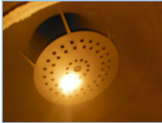
Fig. 1. Flue Gas Diffuser at top of GCT
