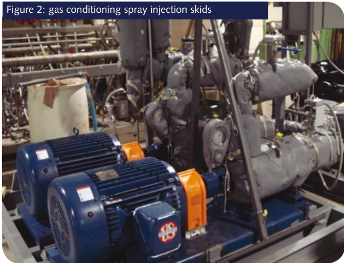
Figure 2: gas conditioning spray injection skids
